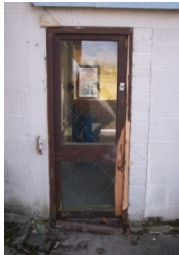
Door broken by thieves
